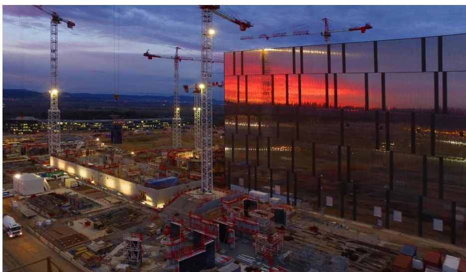
Recent picture of the ITER construction site, with the setting sun reflected on the assembly hall.
