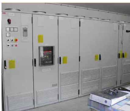
10 Multidrive panels for the downhill conveyor [2]
