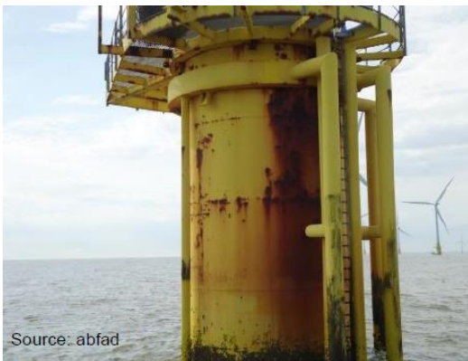
Figure 1 Transition piece (expected to be protected from corrosion) of which the corrosion protection system has become damaged.
